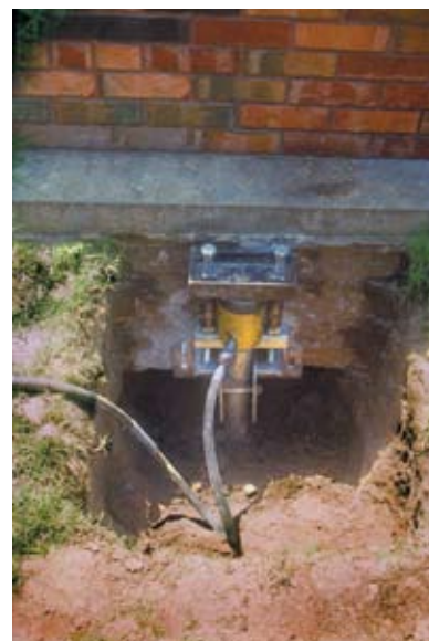
Hydraulic jack pushes down on helical pile shaft and up on foundation held in bracket. After jacking, nuts on top of T-pipe secure the load. Then, jack and plate above are removed to complete installation.
